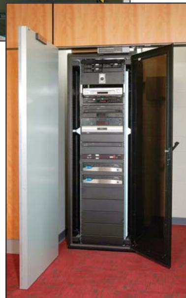
(Top) The communications rack inside the multi-use building incorporates the volume control and AM/FM tuner and CD player connected to the platform and whole building paging system. (Above) This audio-video cabinet is in the side room of the community room.
