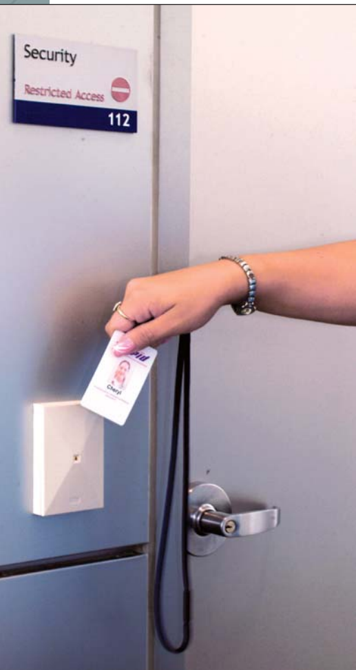
Proximity identification cards cover employee access doors in the multi-building facility.
