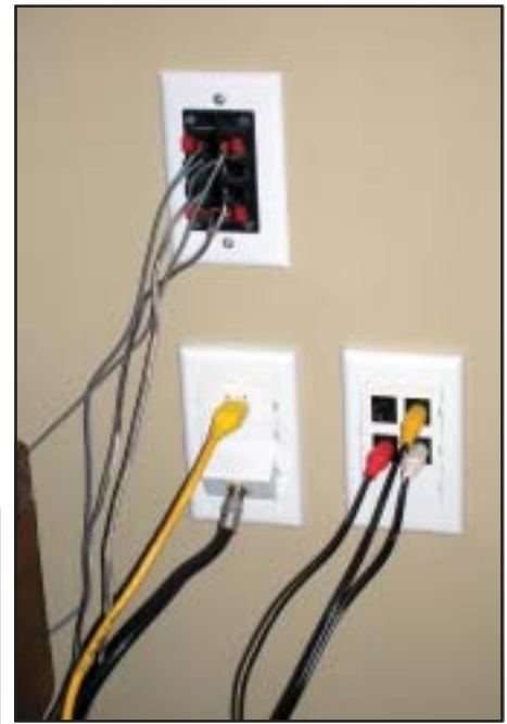
Combining audio/video and data into the same faceplates has applications in residential installations as well as educational buildings.
