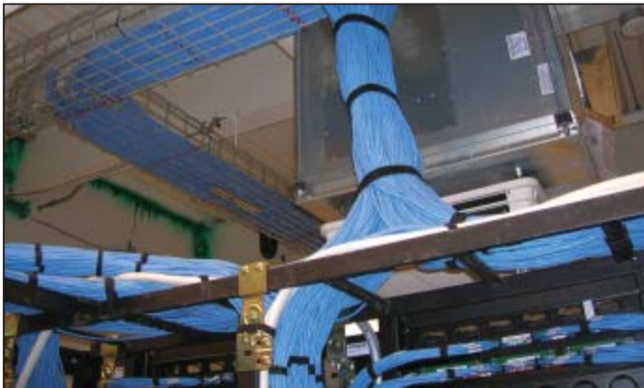
Any of these Cat6 cables that route back to the panels in the communications room could be used for transmitting video and audio signals between classrooms or back to the video distribution headend equipment.
