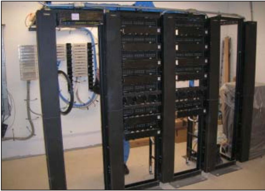
The racks in the main communications room provide a central location for Cat6 cables and fiberoptic cables installed throughout the building.
